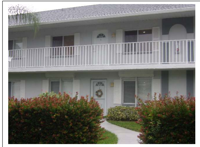
OPENING PROTECTION – Although some unit owners have installed wind-borne debris protection devices, others have not, leaving some of the openings (hinged entry doors, windows & sliding doors) unprotected
