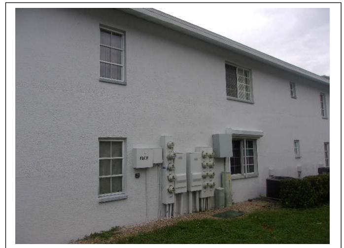
OPENING PROTECTION – Although some unit owners have installed wind-borne debris protection devices, others have not, leaving some of the openings (hinged entry doors, windows & sliding doors) unprotected
