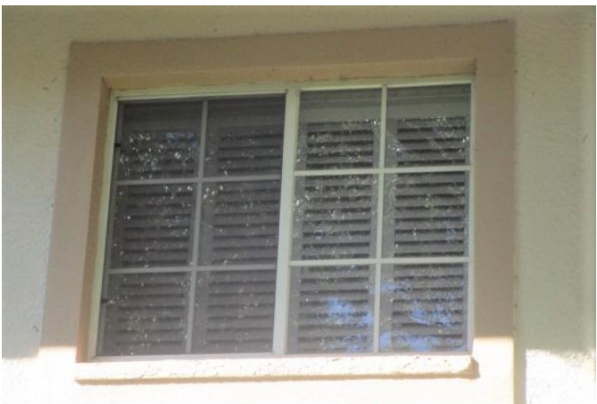
#7) opening protection: some windows are non impact
