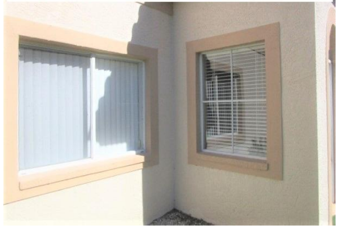
#7) opening protection: non impact windows
