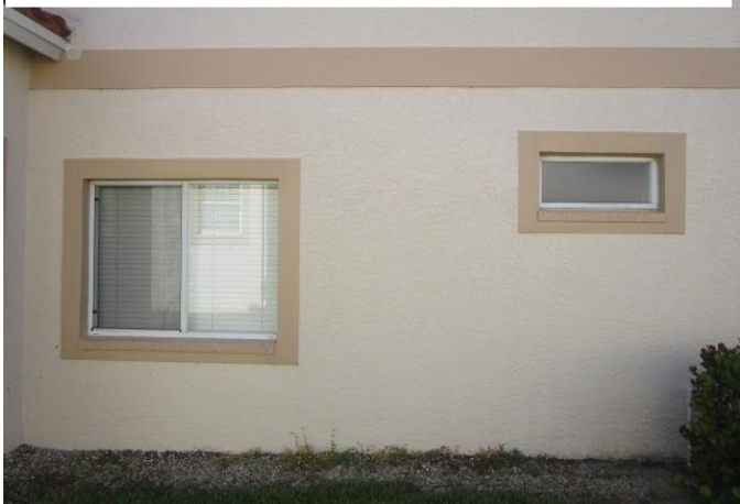
#7) opening protection: non impact windows
