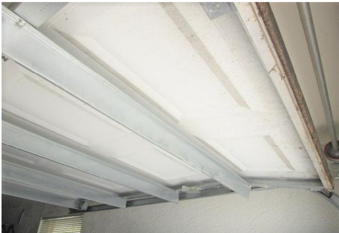
#7) opening protection: non impact garage doors
