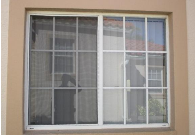
#7) opening protection: non impact windows
