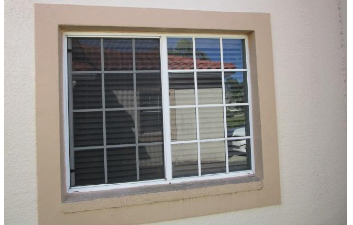
#7) opening protection: non impact windows
