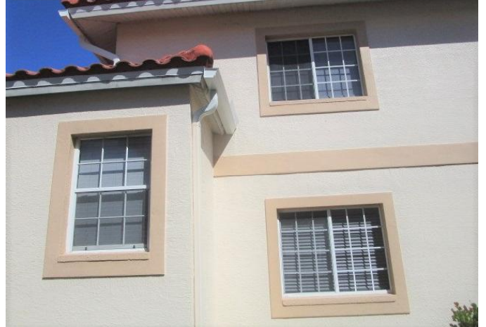
#7) opening protection: non impact windows
