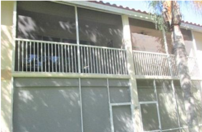
#7) opening protection: non impact rear sliders- some w/roll down shutters
