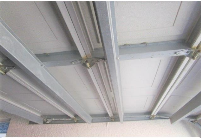
#7) opening protection: non impact garage doors
