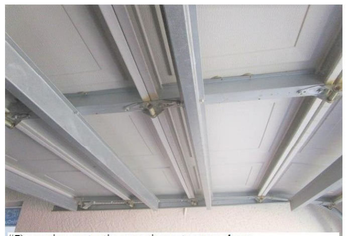
#7) opening protection: non impact garage doors
