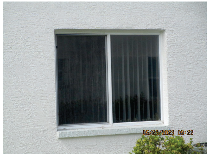
non impact windows- no hurricane protection
