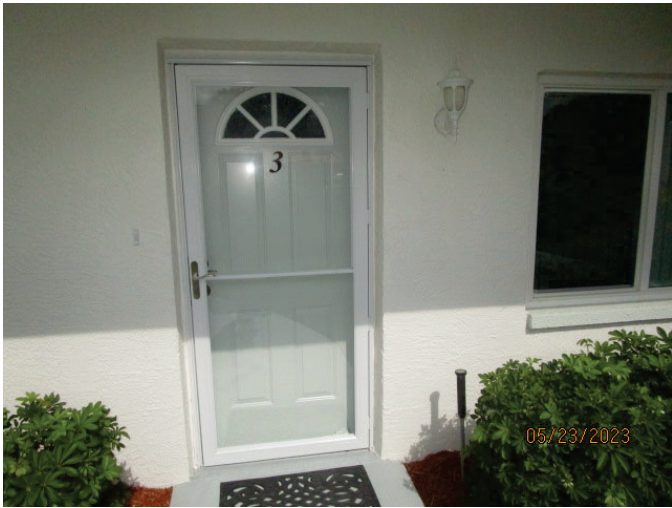
opening protection: non impact front doors
