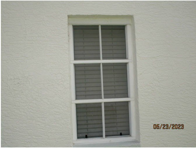
non impact windows- no hurricane protection
