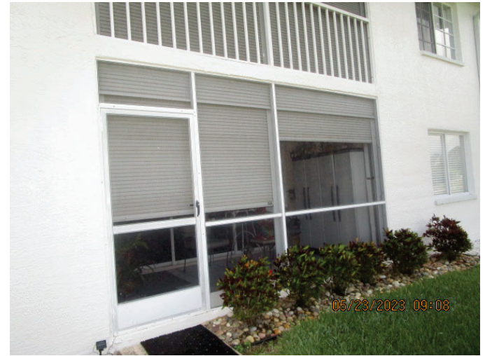
rear porches have roll down shutters (not impact verified)
