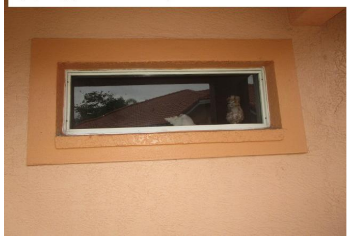
#7) opening protection: non impact windows
