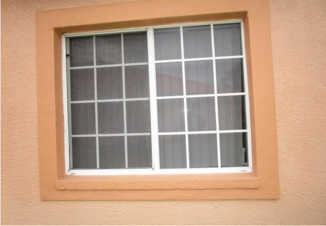
#7) opening protection: non impact windows
