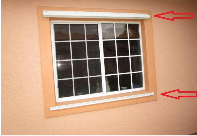
#7) opening protection: non impact windows w/metal panels
