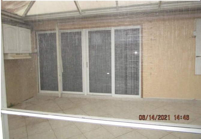
#7) opening protection: impact rated sliders
