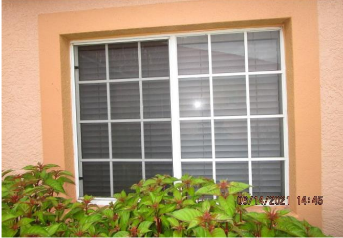
#7) opening protection: non impact windows
