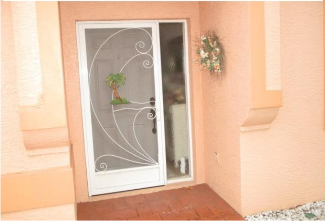
#7) opening protection: metal clad door w/non impact sidelite
