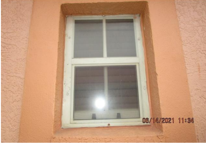
#7) opening protection: non impact windows some w/acrylic
