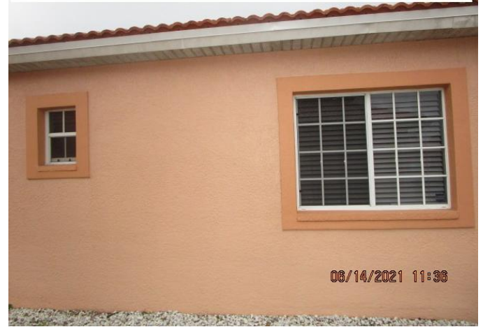
#7) opening protection: non impact windows
