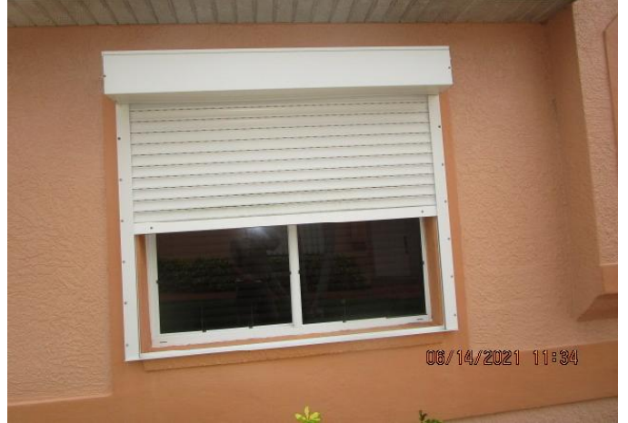
#7) opening protection: non impact windows some w/roll downs
