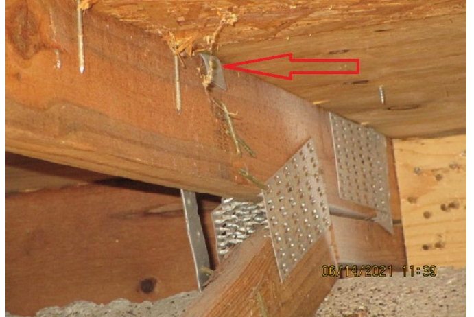
#4) roof to wall attachment: single wraps- opposite view
