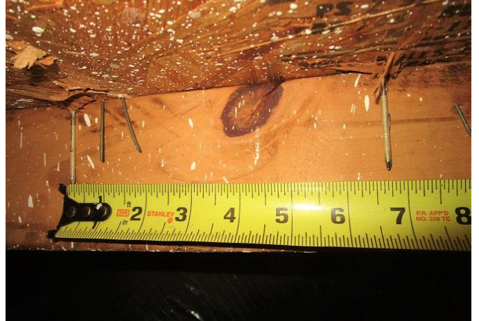
#3) roof deck attachment: 8d nail spacing
