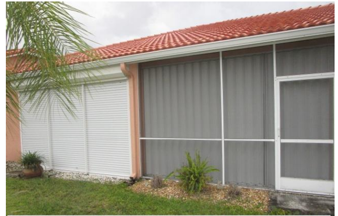
#7) opening protection: non impact windows, doors & sliders all with some form of protection (metal panels or roll downs)
