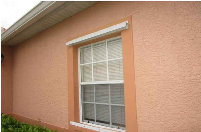
#7) opening protection: non impact windows, doors & sliders all with some form of protection (metal panels or roll downs)
