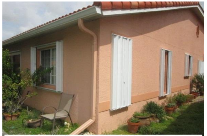
#7) opening protection: non impact windows some w/shutters some without protection
