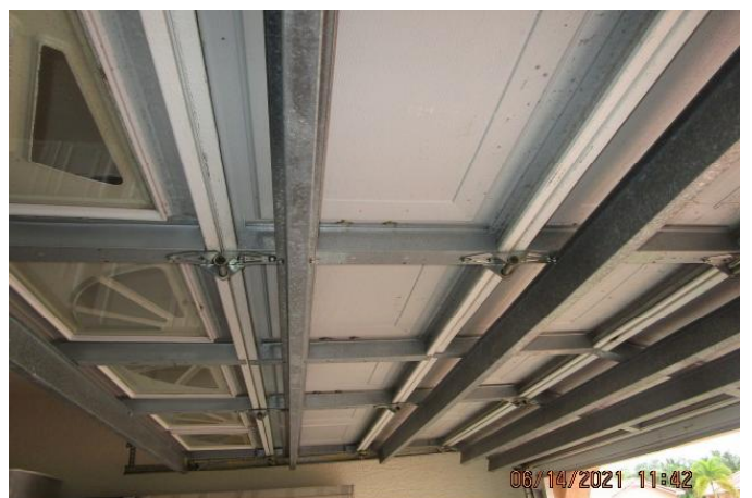
#7) opening protection: wind rated non impact garage doors
