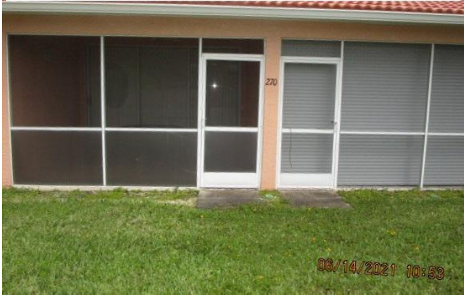
#7) opening protection: non impact rear sliders 1 w/roll down shutters & 1 with no protection
