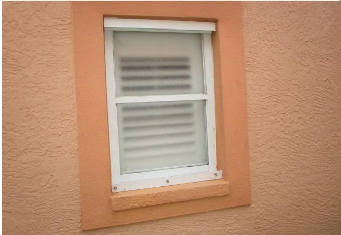
#7) opening protection: non impact windows w/metal panels
