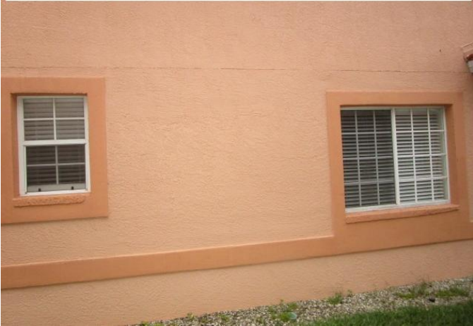
#7) opening protection: non impact windows
