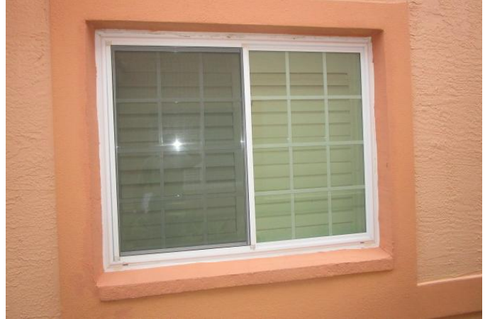
#7) opening protection: non impact windows
