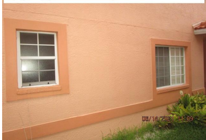
#7) opening protection: non impact windows
