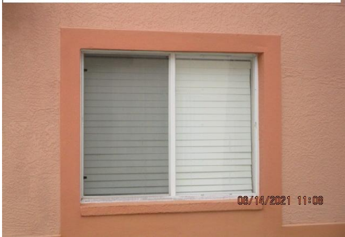
#7) opening protection: non impact windows
