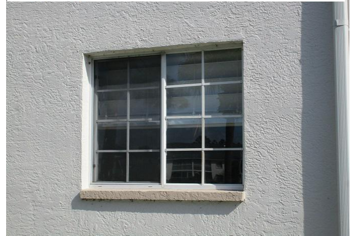
#7) opening protection: non impact windows
