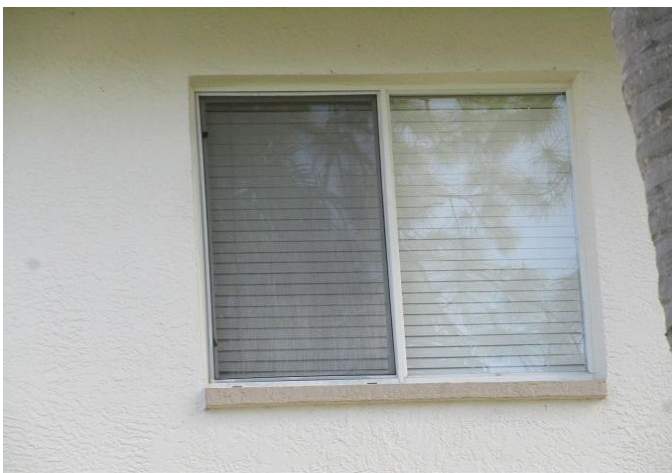
#7) opening protection: non impact windows
