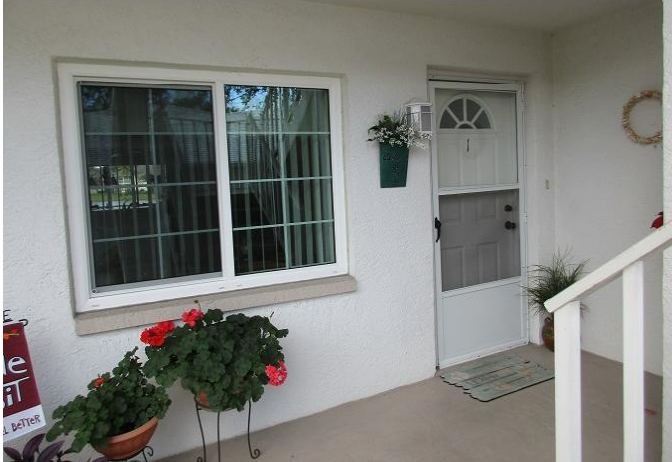
#7) opening protection: non impact front entrance
