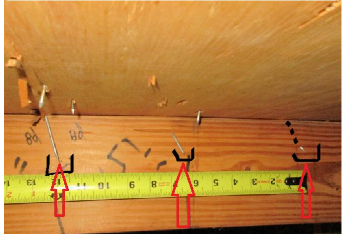
#3) roof deck attachment: 8d nail spacing
