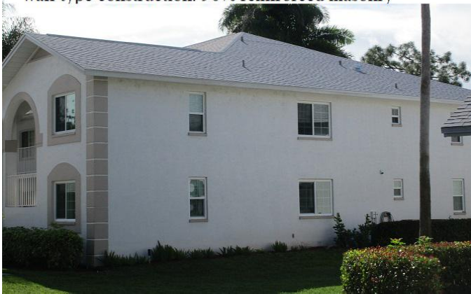
#5) roof geometry: HIP style roof *42' Front gable vs 480' total roof perimeter or less than 10% **wall type construction: 90% reinforced masonry
