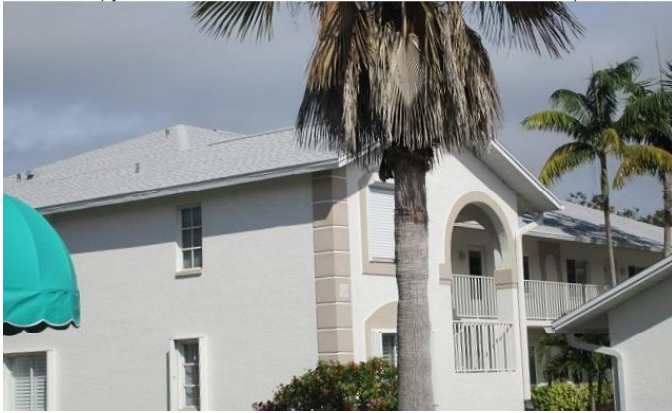
#5) roof geometry: "other" (gable) style roof *42' front gable vs 376' total roof perimeter or more than 10% **wall type construction: 90% reinforced masonry
