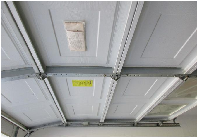
#7) opening protection: non attached garage w/non impact door
