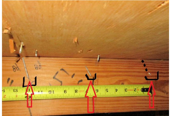
#3) roof deck attachment: 8d nail spacing
