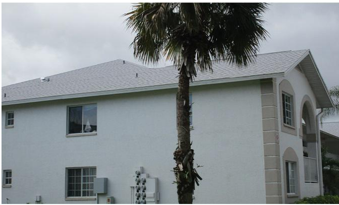
#5) roof geometry: HIP style roof *42' Front gable vs 480' total roof perimeter or less than 10% **wall type construction: 90% reinforced masonry
