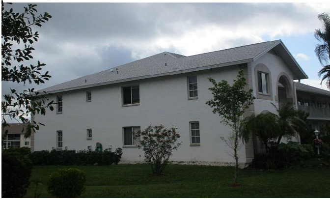
#5) roof geometry: HIP style roof *42' front gables vs 480' total roof perimeter or less than 10% **wall type construction: 90% reinforced masonry
