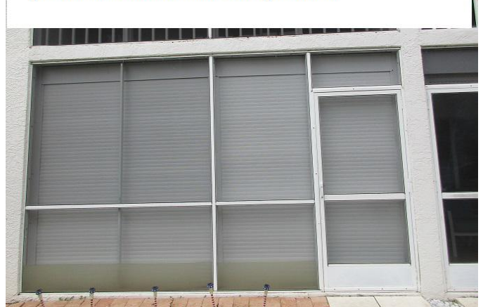
#7) opening protection: non impact sliders- some with storm protection & most without storm protection
