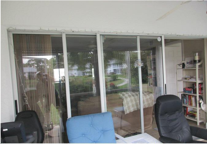
#7) opening protection: non impact sliders (some w/roll down shutters)
