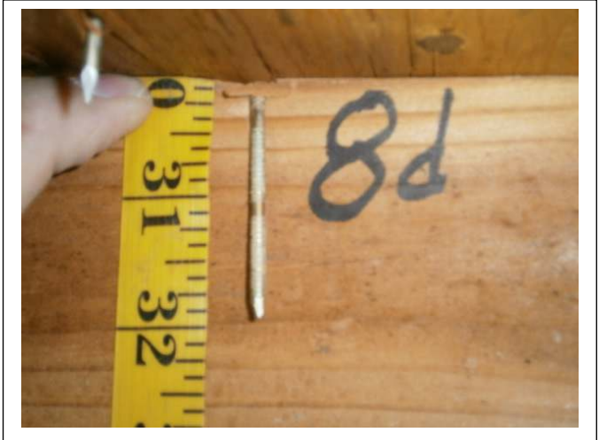
ROOF DECK ATTACHEMNT – 8d ring shank nails added in 2022
