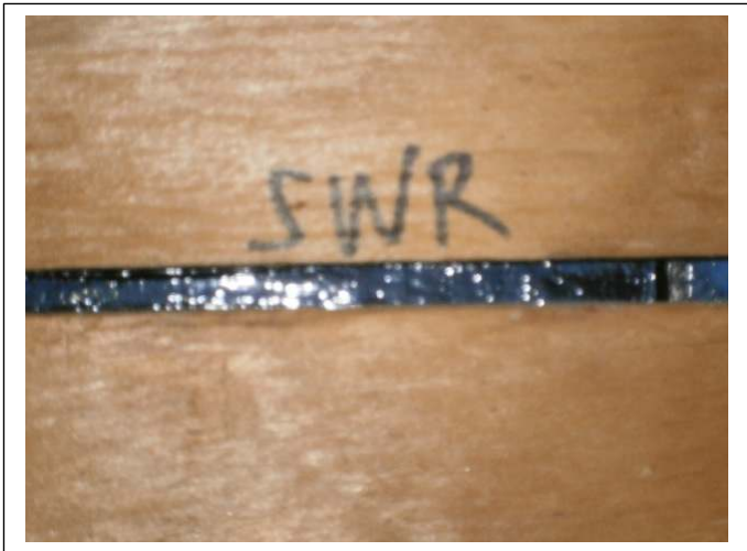
SECONDARY WATER BARRIER – A polymer adhesive (peel & stick) SWR Barrier was installed on the entire roof deck in 2022
