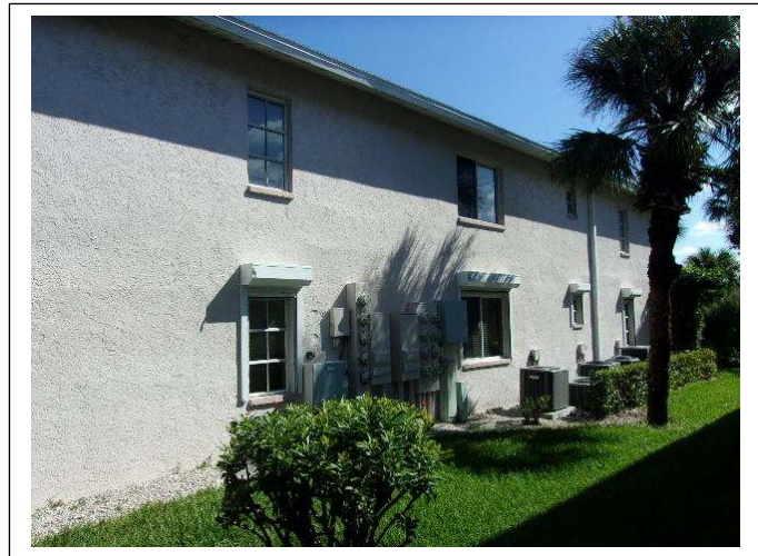
OPENING PROTECTION – Although some unit owners have installed wind-borne debris protection devices, others have not, leaving some of the openings (hinged entry doors, windows & sliding doors) unprotected
