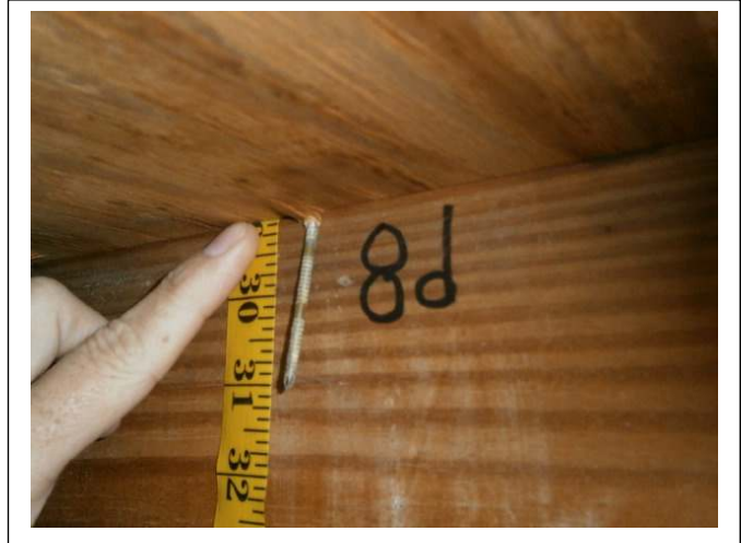
ROOF DECK ATTACHEMNT – 8d ring shank nails added in 2019
