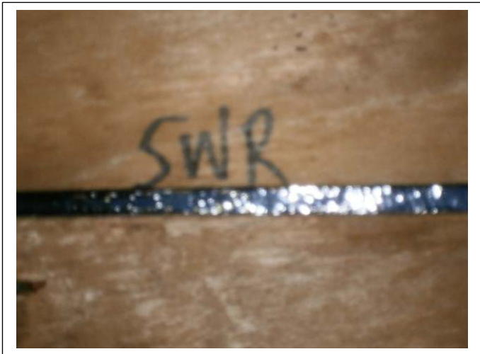
SECONDARY WATER BARRIER – A polymer adhesive (peel & stick) SWR Barrier was installed on the entire roof deck in 2019
